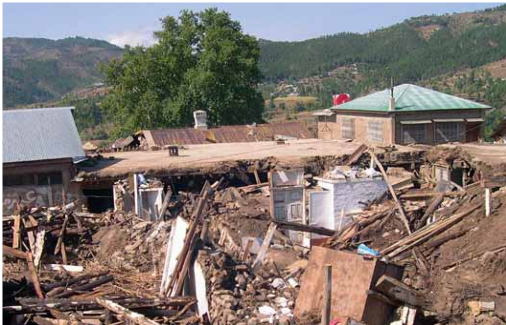
Earth Quake in Pakistan 2005: Destruction in Baddal town, Mansehra district, Photo: EC/ECHO/Nick Bridger
